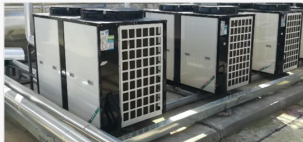
The demonstration project of VI-ASHP installed.
