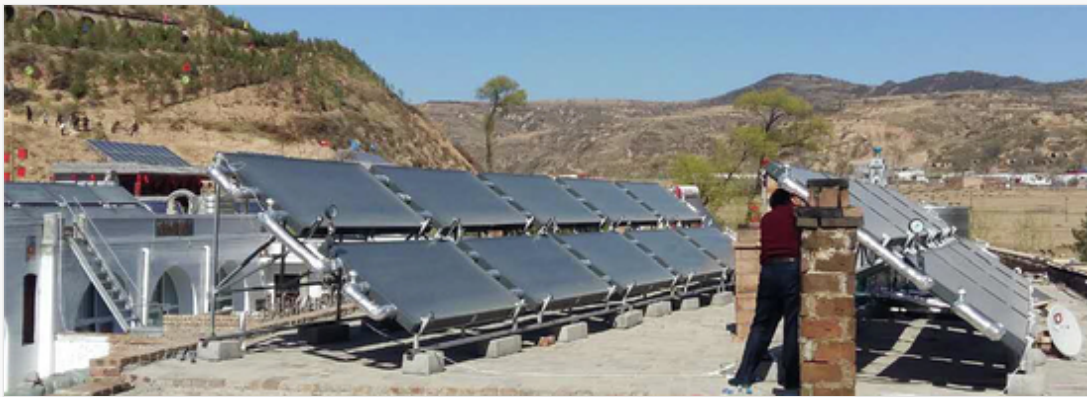
The demonstration of the solar energy systems installed at the demonstration site.
