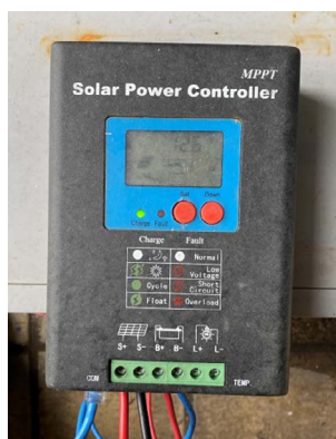
(c) PV panel data collector
