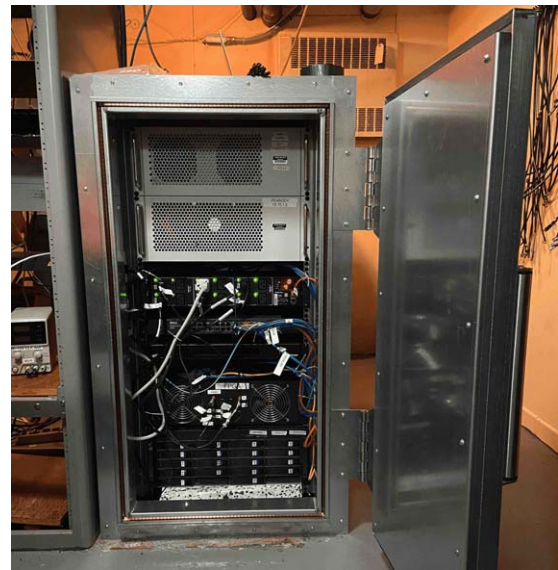
Figure 5. RF-shielded rack located in the main control room at ARO. The rack includes (from top to bottom): controller node, analysis node, power distribution unit (PDU), main switch, GPS unit, ICE/FPGAs, and recording node.
