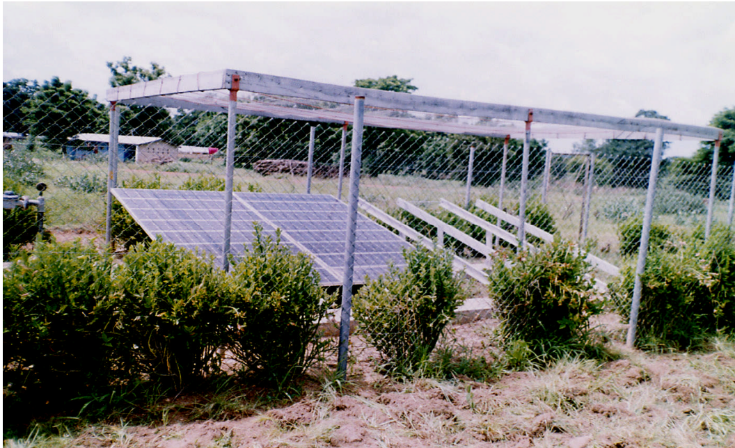
Plate 5.3 Solar PV water pump system at Wechiau in Wa West district
