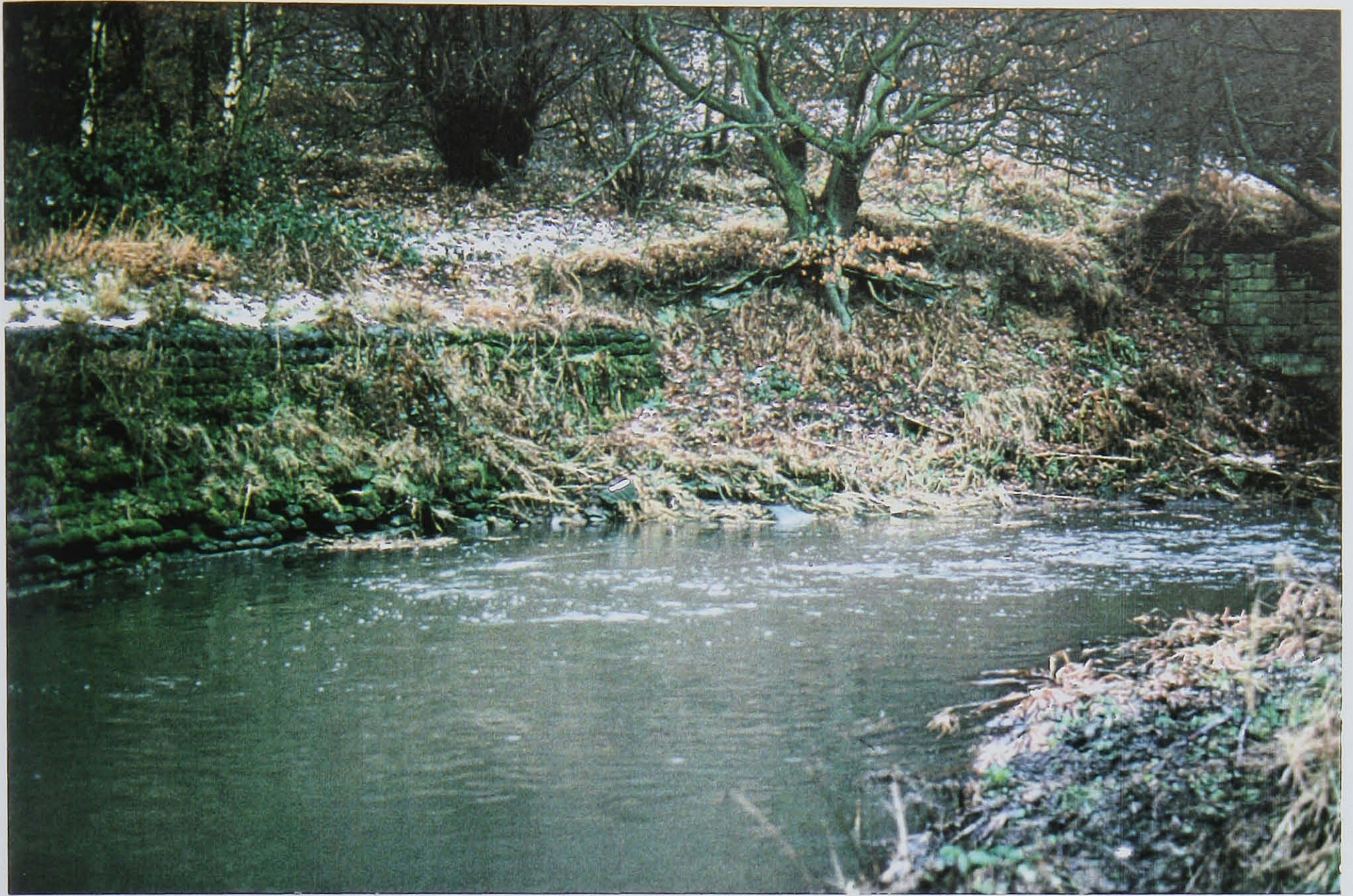
Plate 3. The River Dearne at Cudworth Common with ageing flood defence walls and eutrophicating waters.
