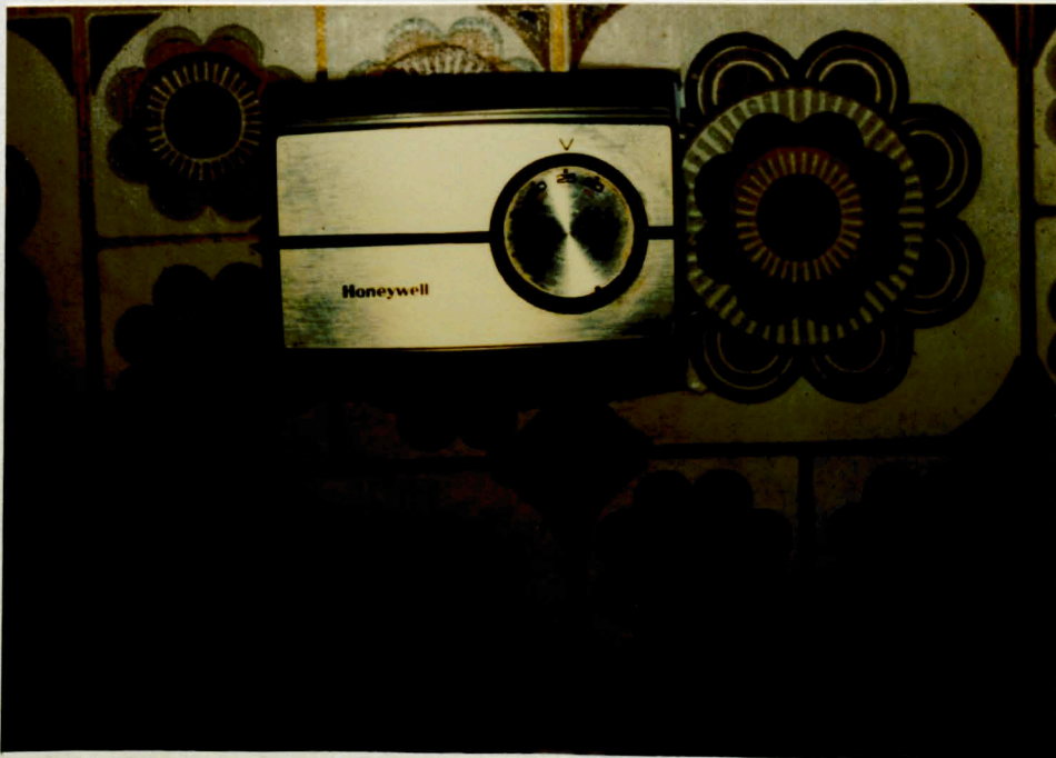
6:6 The room thermostat in the gas homes
