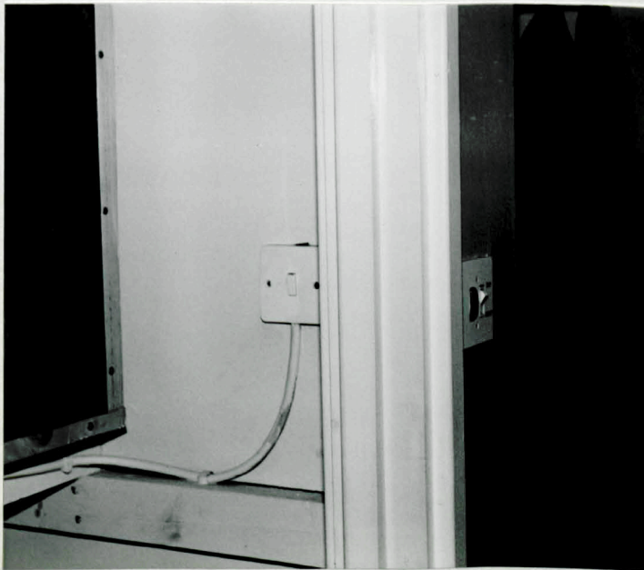
4:13 Mrs D's two water switches: on the right the Day/Night control, on the left the immersion heater switch
