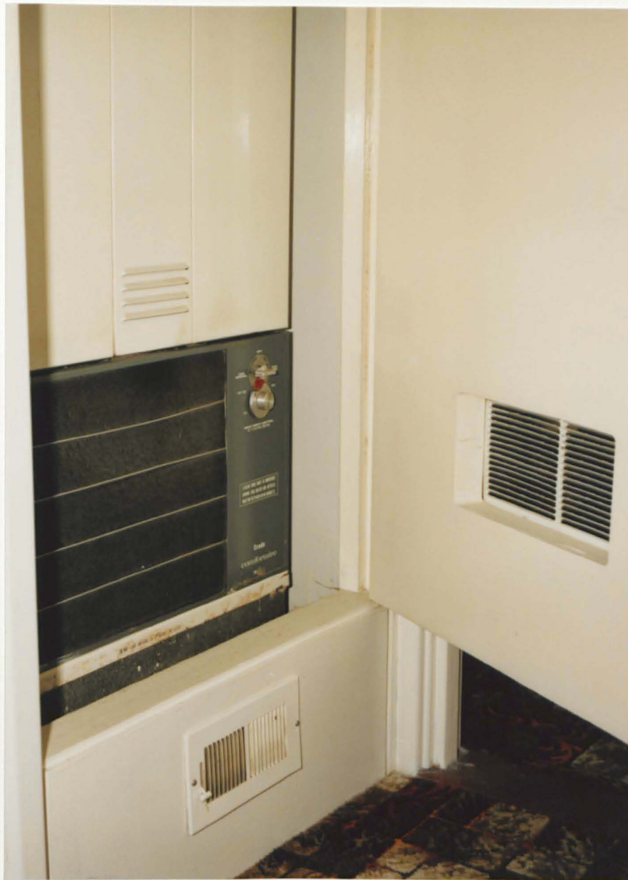
2:2 The Electricaire storage heating unit
