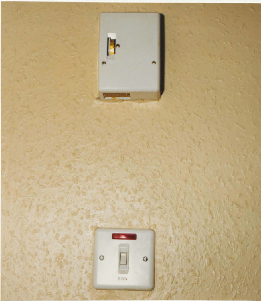
2:6 Room thermostat and fan switch
