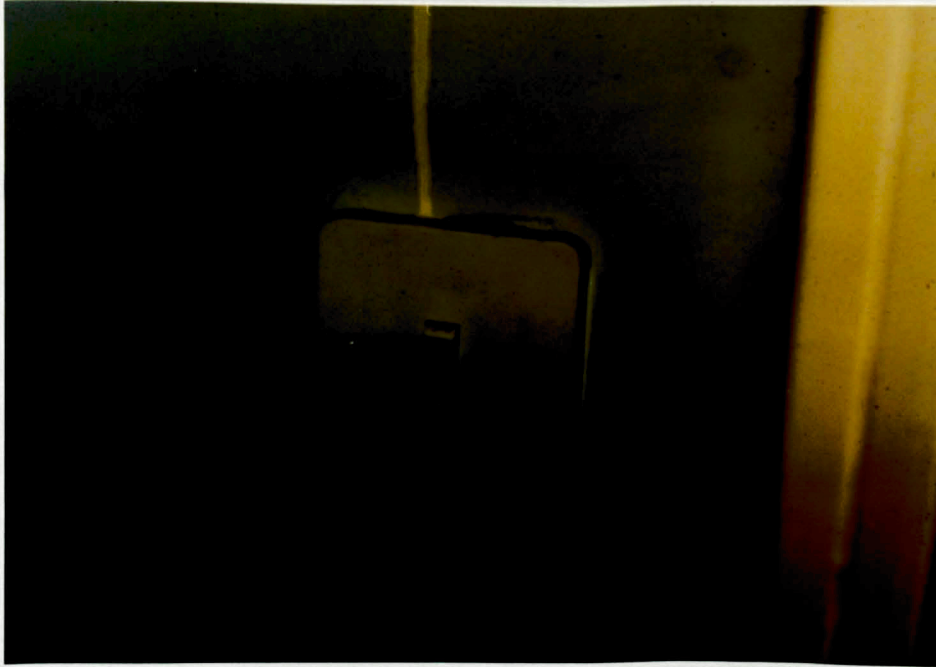
4:12 The switch by Mrs D's immersion heater
