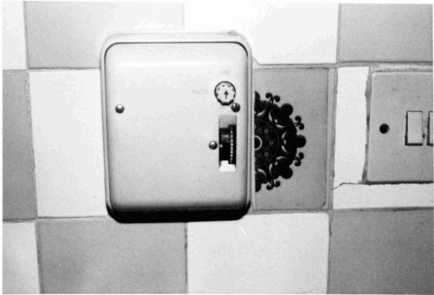
6:7 A thermostat controlling underfloor heating
