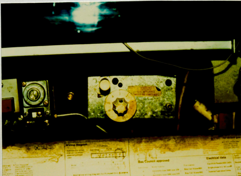
6:3 The uninformatively labelled boiler thermostat
