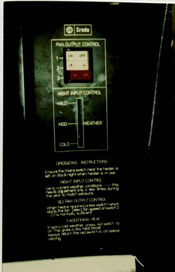
4:10 The rocker switches that Mrs M put off each night
