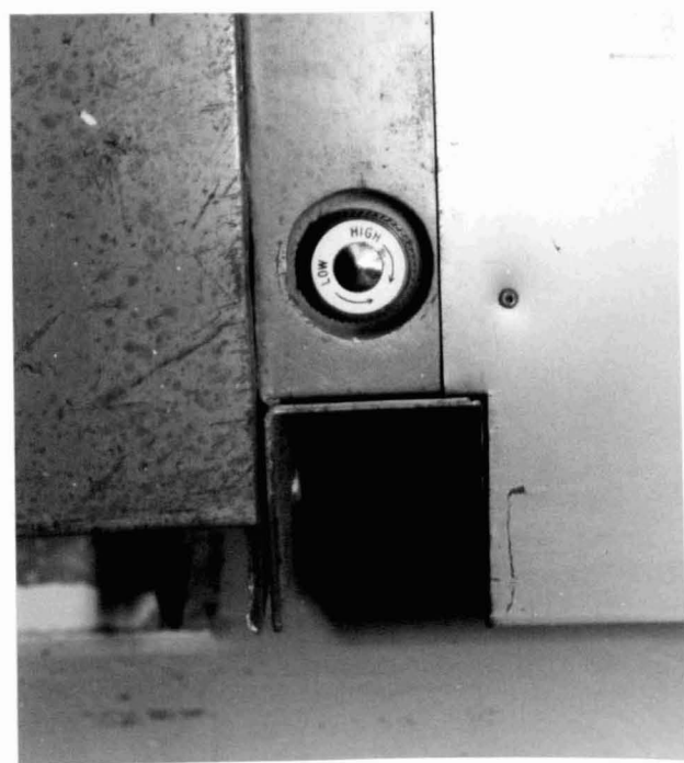
4:6 The insufficiently labelled charge control in Mrs L's house
