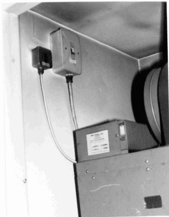
4:4 The switches on the wall above the heating unit in Mrs L's house
