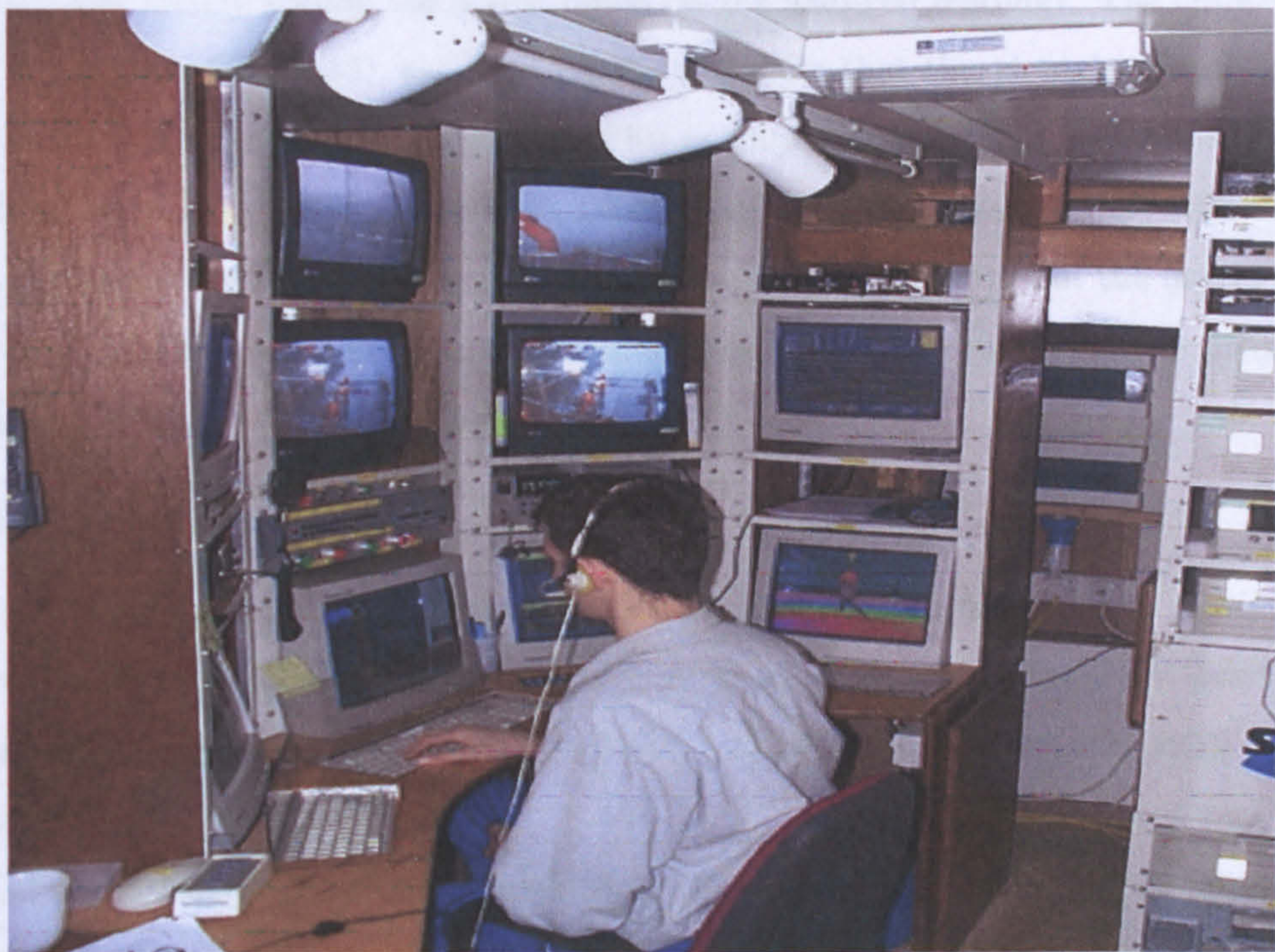
Figure 9.10: WFM implementation in crane control cabin (bottom right monitor)
