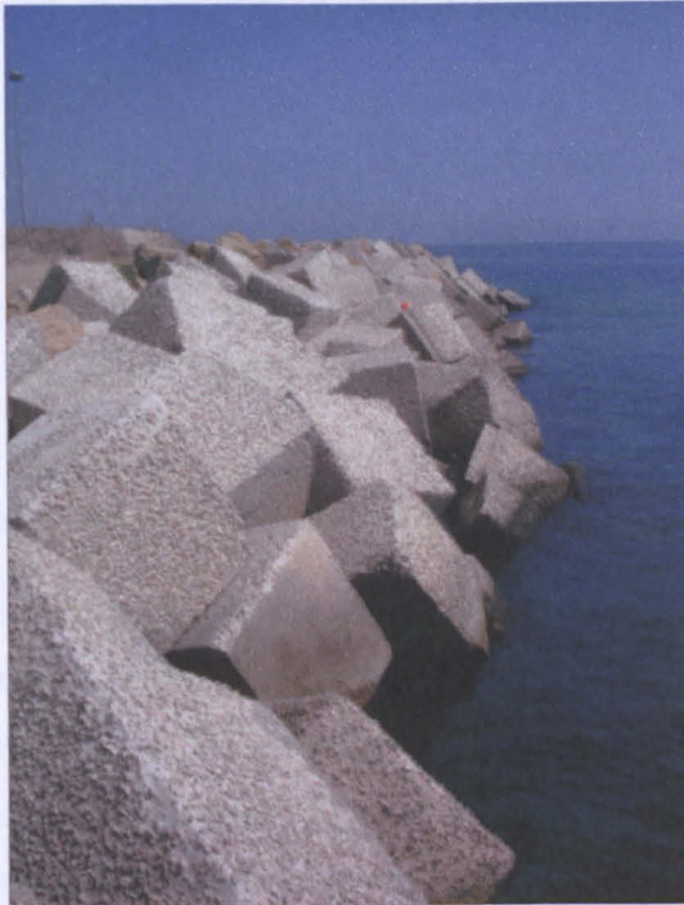
Figure 7.2: Photograph of blocked harbour wall at low tide
