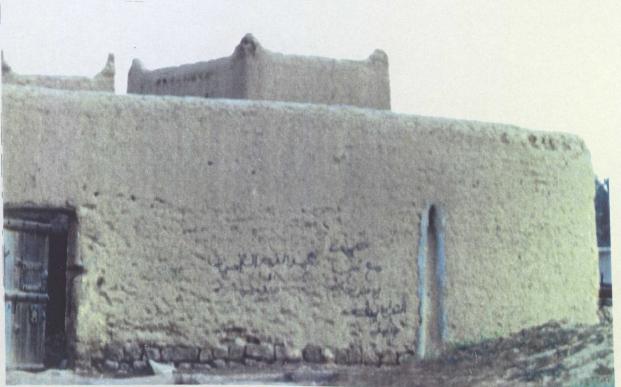
b) Mud House in Hwylan, still in reasonable condition but no longer occupied
