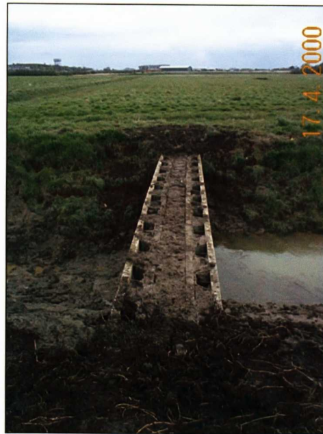
Figure 2.15 The dam installed within the drainage ditch running to the north of the archaeological enclosures. The dams are approximately 0.5 m in width.
