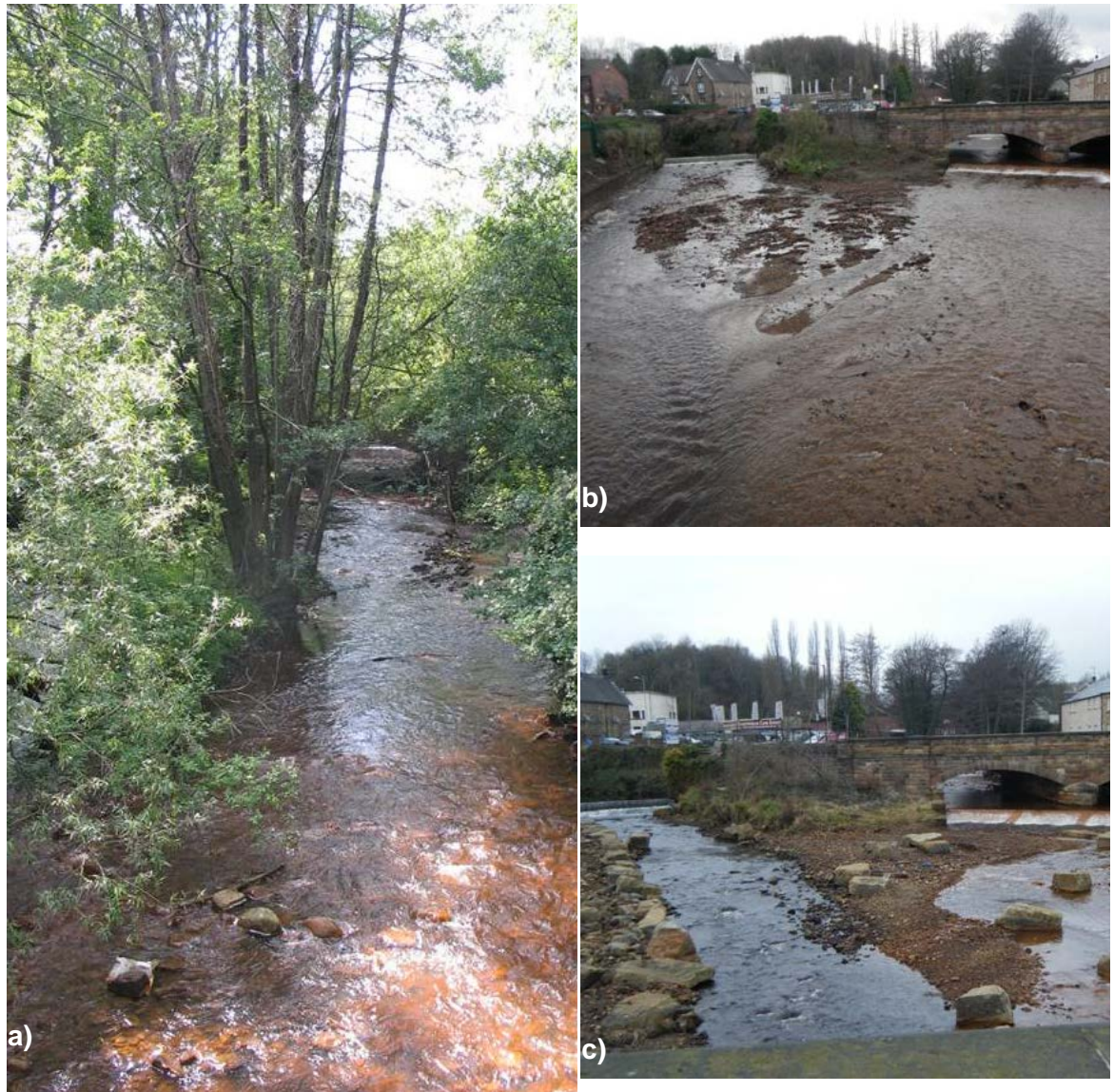
Figure 4.3. Malin Bridge a) before flood defence work (2009), b) after flood defence work (2009) and c) after channel re-profiling (2011), riffle instalment and boulder placement.
