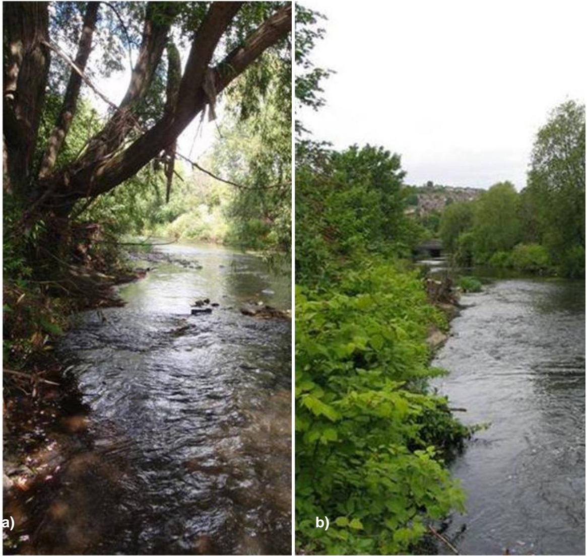
Figure 4.18. Photograph of Brightside before (a) and after (b) channel clearance works took place.
