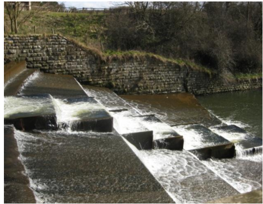
b) Newly installed fish pass on the Sea Cut just before conjoining with Scalby Beck
