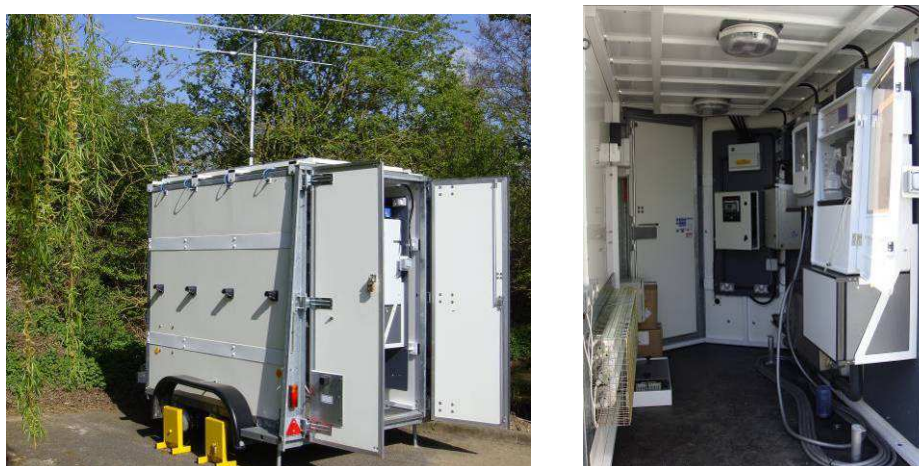
Figure 1.2: Example of shed housing instruments at the river Cut [16]
