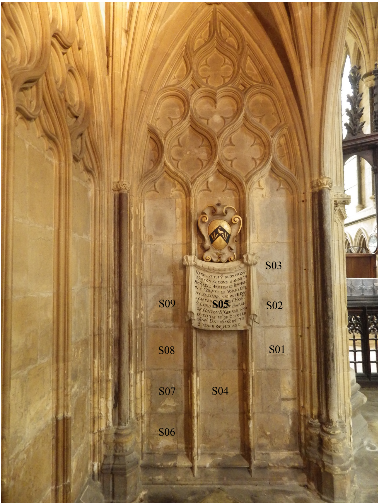
Figure Appendix 2.4: The numbered stone blocks on the north return bay which show evidence of graffiti
