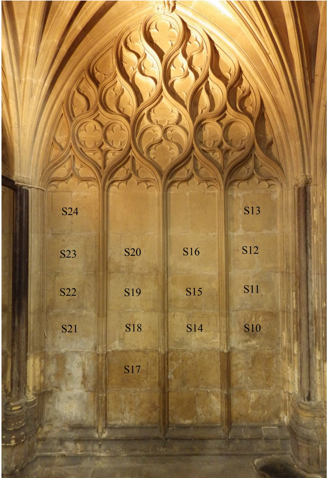
Figure Appendix 2.1: The numbered stone blocks on the right-hand bay which show evidence of graffiti
