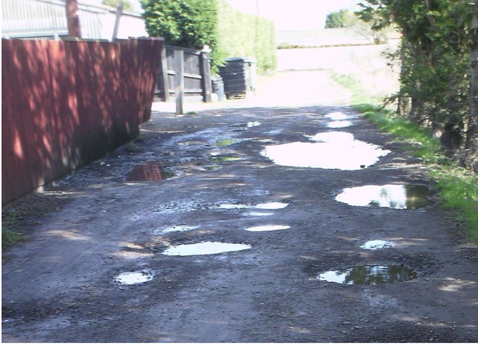
Figure 9a: Potholes in road to temporary unauthorised development, photographed by B. Parnell-Berry (2010).
