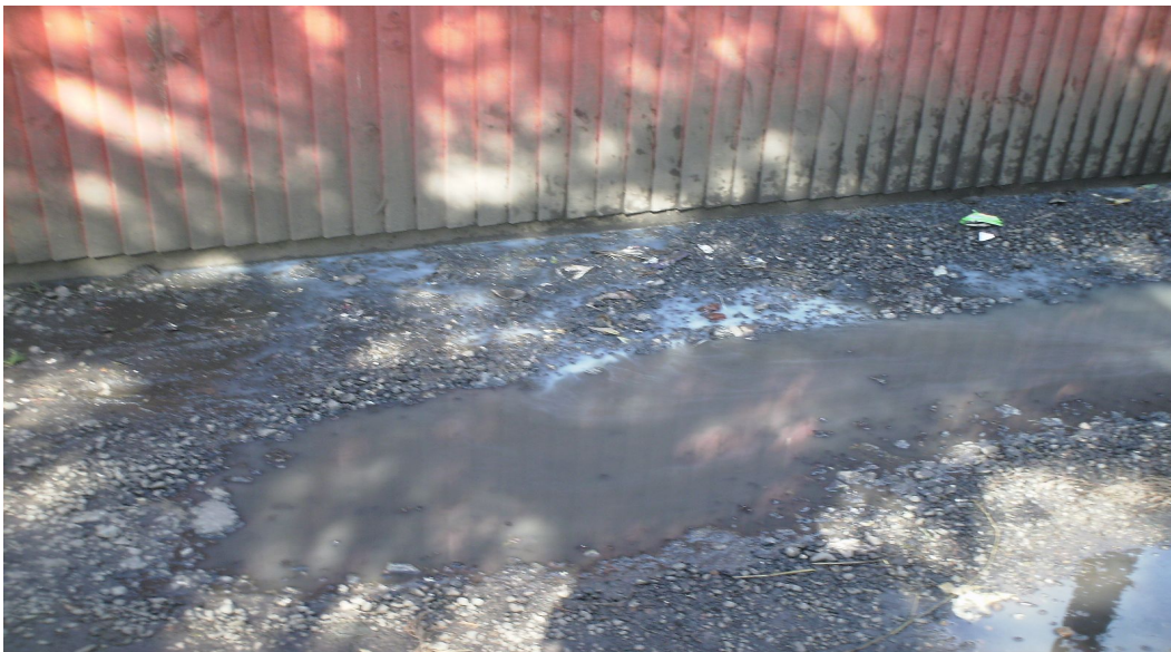
Figure 9b: Raw sewage on temporary unauthorised development, photographed by B. Parnell-Berry (2010).
