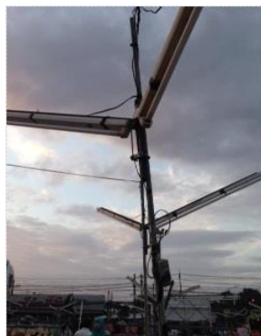
Figure 42 Lights are installed in every unit
