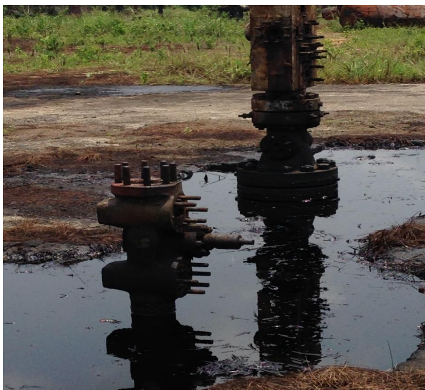
Figure 16: Crude-Oil Leakage at Omu Village
