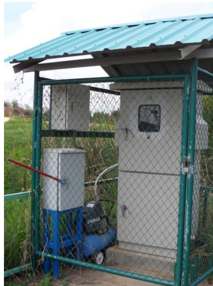
Figure 30 Online system for monitoring COD and BOD (Source: author)
