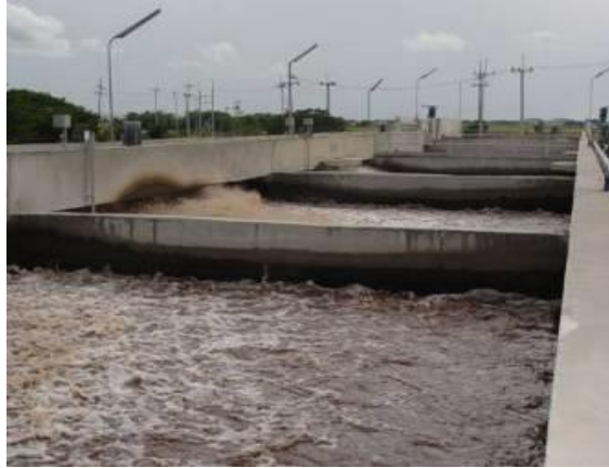
Figure 38 Oxidation tank (Source: author)
