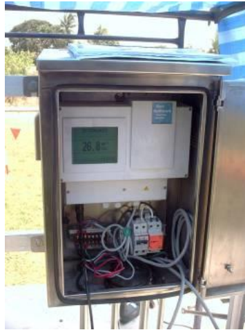
Figure 41 COD and BOD monitoring and reporting equipment (Source: author)
