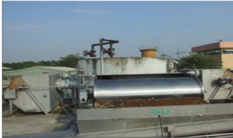
Figure 35 Drum screen (Source: the company provided to the author)
