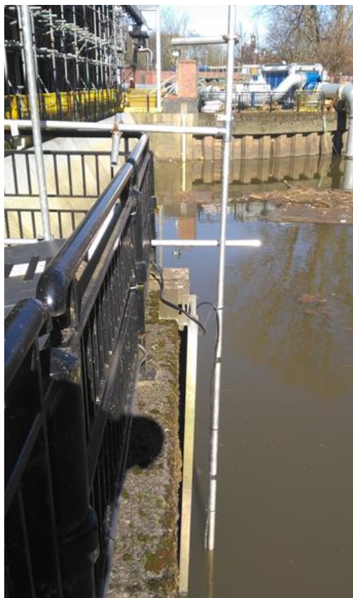
Figure 21 DIDSON installation at Foss
