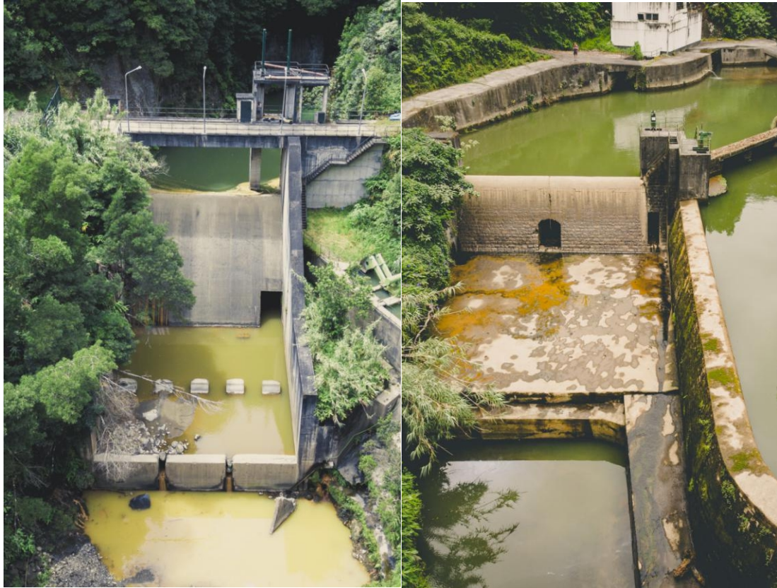
Fig. 14. Two hydroelectric dams intersecting Ribeira Quente at 1530 m (left) and 4550 m (right) from the ocean.
