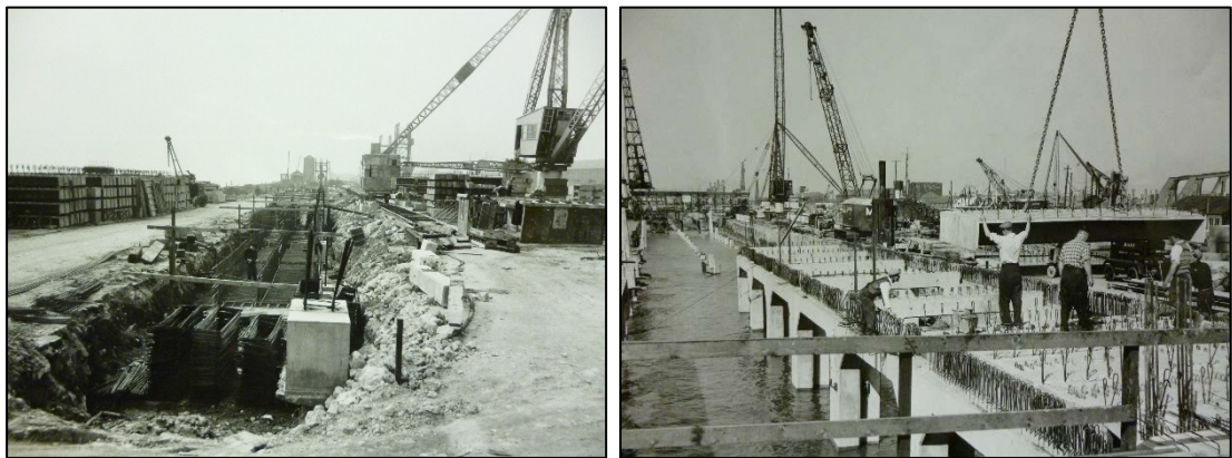
Figure 10: Photographs showing the new Riverside Quay under construction in 1957, some 16 years after the destruction of the old quay. (Photographs courtesy of Associated British Ports).
