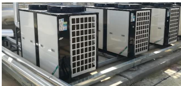
Fig. 8-2 Demonstration of installed VIHR-ASHP
