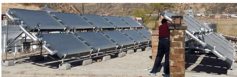
Fig. 8-1 Demonstration of installed solar thermal collector
