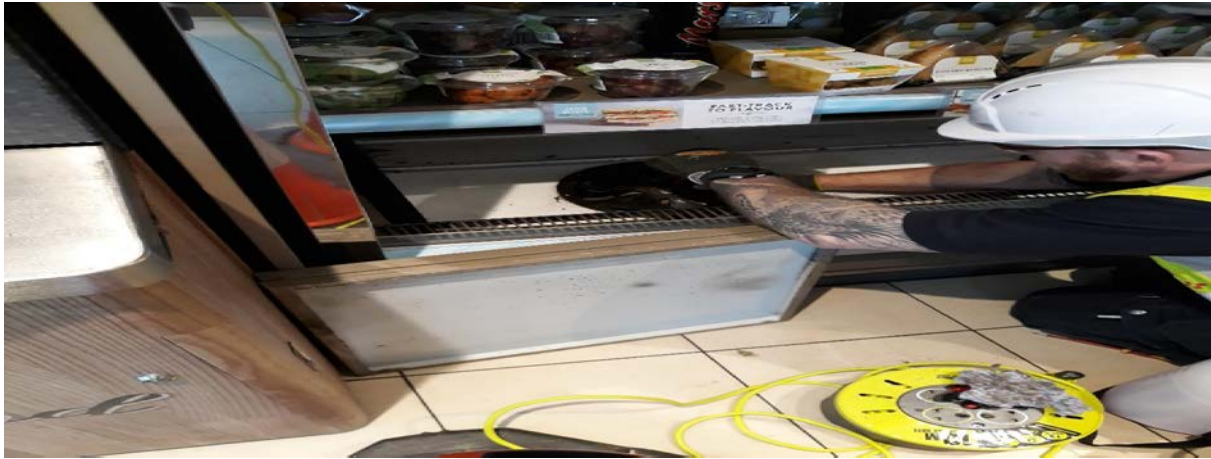
Fig 5 Fridge clean pre planned maintenance as part of the FMC contract
