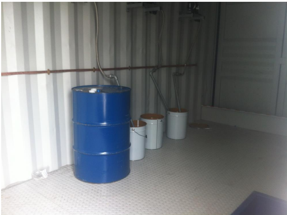
5.12: Solvent pumping system and solvent barrel.
