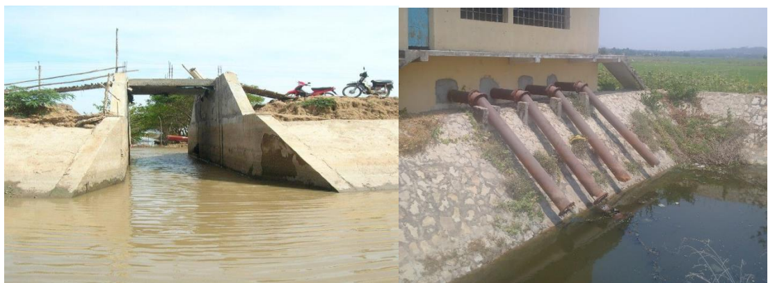
Figure 4-6. A recent decrease in water levels in the upper part of VMD has resulted in reduced efficiency of infrastructure elements like pumps and sluice systems. The photo took place in 2019 and provided by SIWRR
